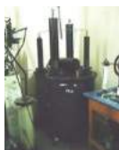
Fig. 1. 75/150 kV Siemens-Schuckert transformer at HV lab of Lviv Polytechnics from 1913
